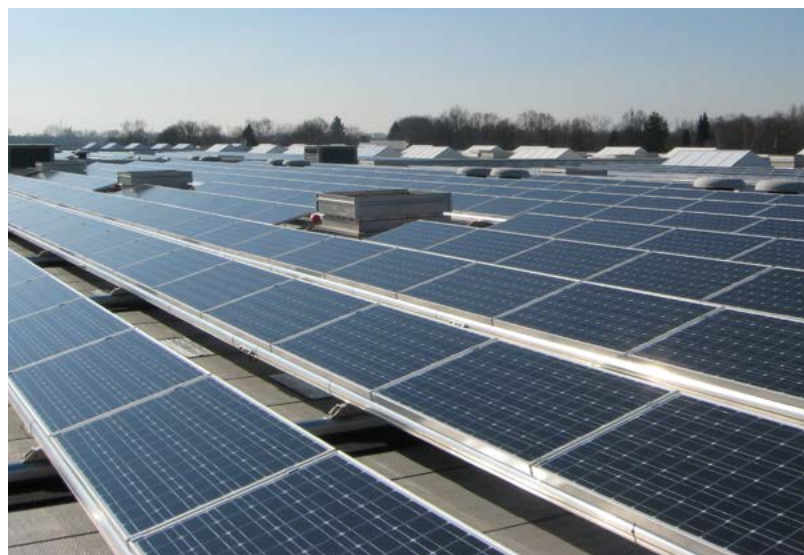
Photovoltaic cells on the company building
