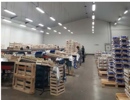
LED lamps in sorting rooms
